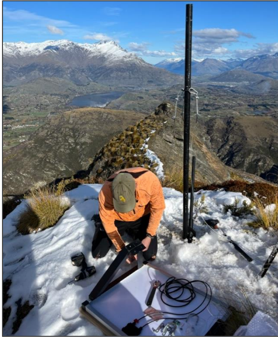
Figure 9 - Mounting solar panel brackets to the solar panel for the Radio Comms Tower.
