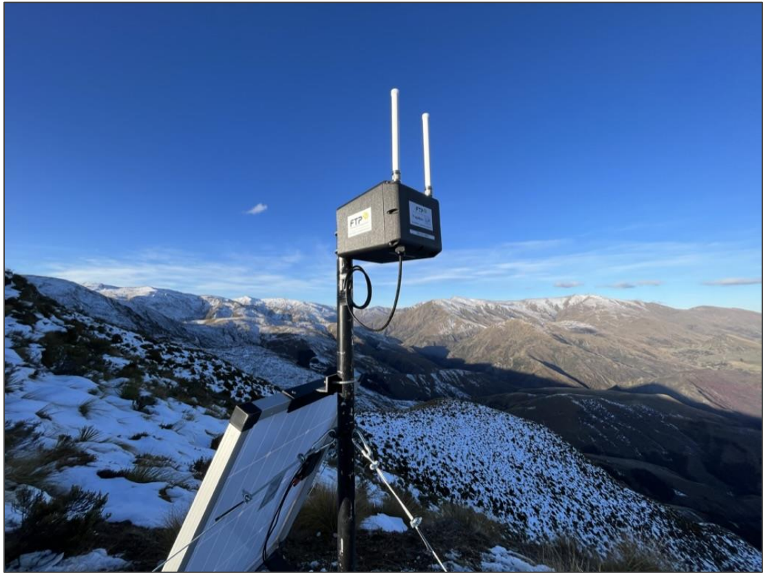
Figure 12 - Yarn Mesh Gateway on a Yarn Mesh Radio Comms Tower showing guy wires.
