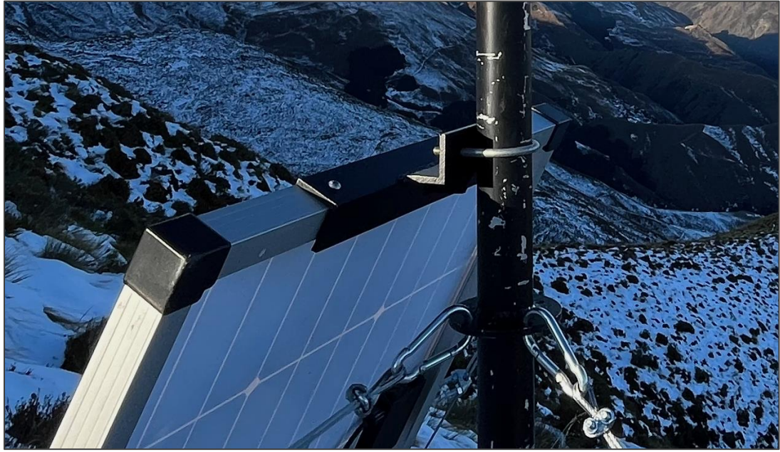
Figure 10 - RCT showing solar panel mount U-bolts and guy wire carabiners.
